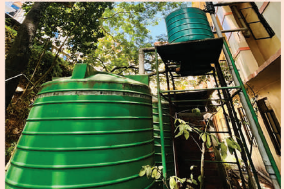
Rain Water & West Water Recycling
